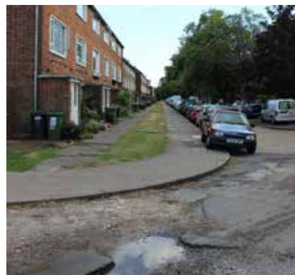
Figure 20: Poor quality streetscape and public realm.
