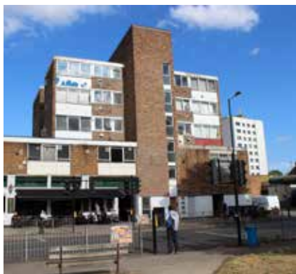
Figure 18: Poor quality building facade.
