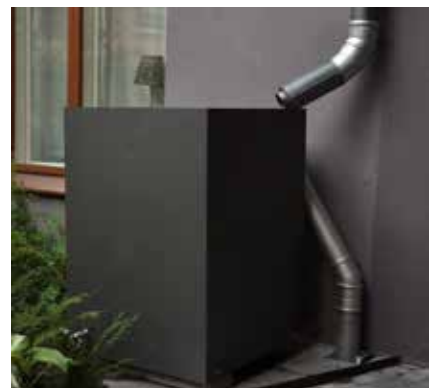
Figure 80: Water harvesting tank.
